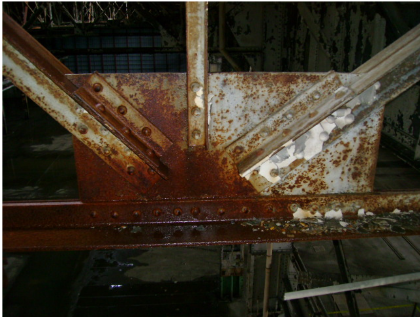
Photo #18: Typical corrosion along bottom chord of roof truss
