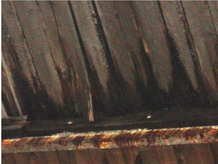
Photo #50: Typical roof deck rotting and deterioration
