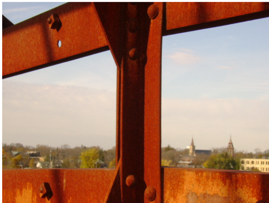
Photo #17: Typical warped apex vertical member in fire damaged region
