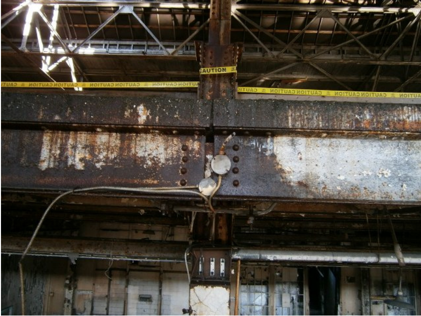
Photo #30: Typical corrosion of steel at mezzanine slab edge
