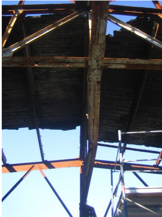
Photo #16: Typical warped tie-truss in fire damaged region
