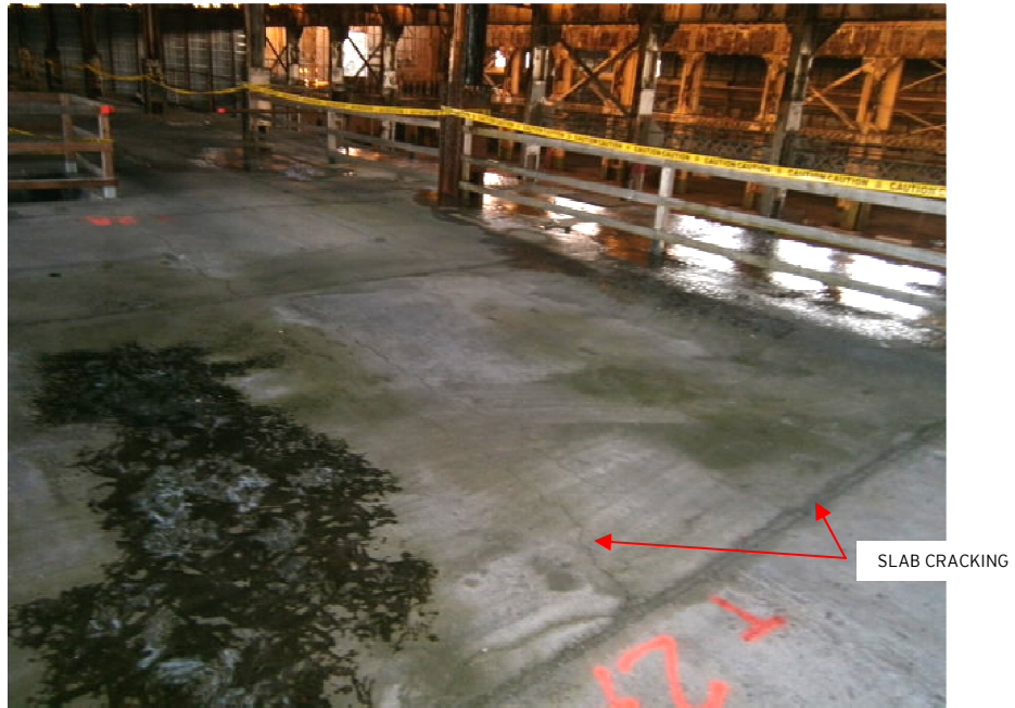
Photo #26: Typical mezzanine slab cracking
