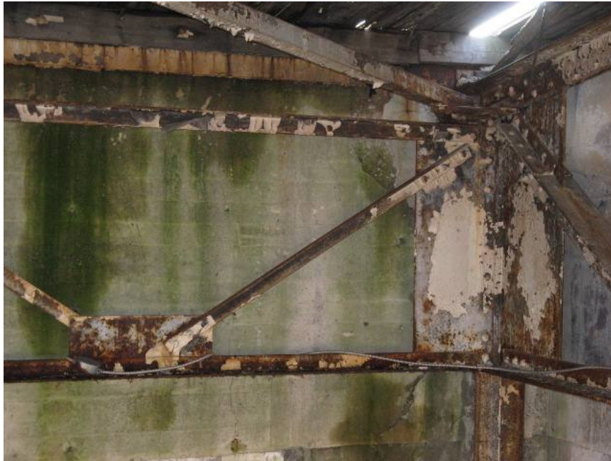
Photo #32: Corrosion at tying truss near grid 'Cs-1'
