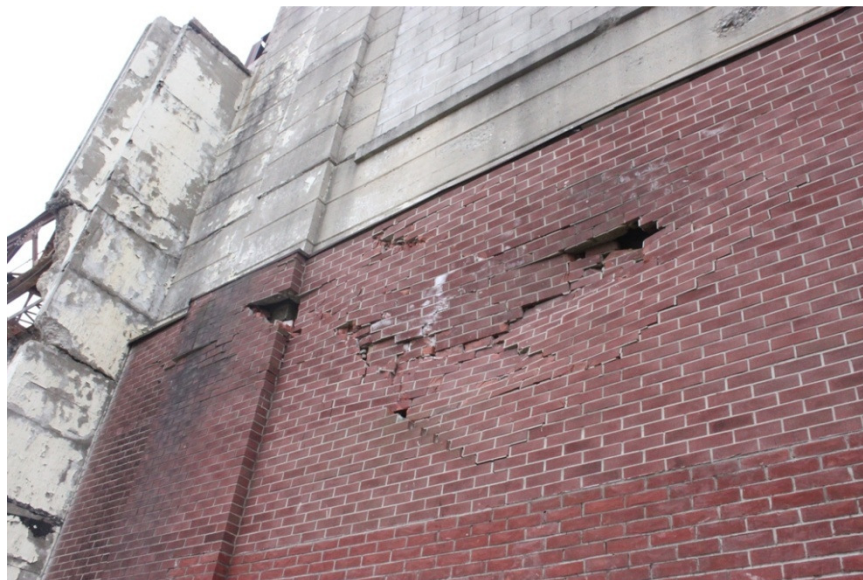
Photo #45: Impact damage and deterioration of exterior brick veneer
