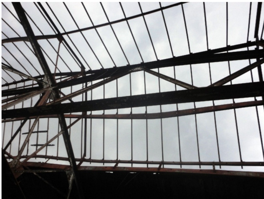
Photo #15: Typical warped purlins in fire damaged region
