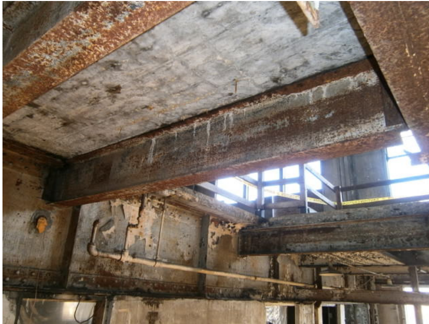
Photo #28: Typical corroded steel and slab soffit deterioration near slab opening
