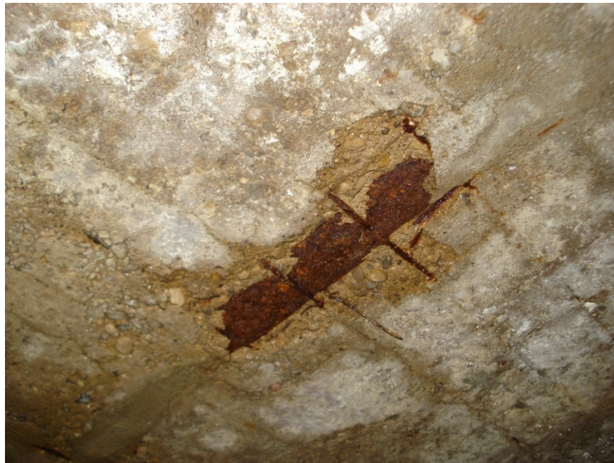
Photo #27: Mezzanine slab soffit delamination and exposed reinforcing steel
