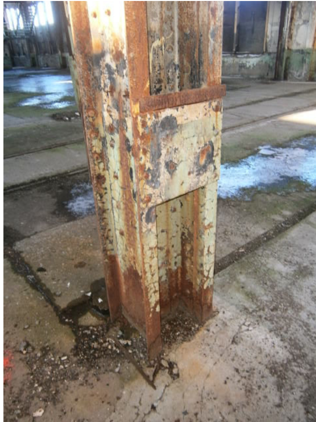
Photo #23: Typical corrosion at column base
