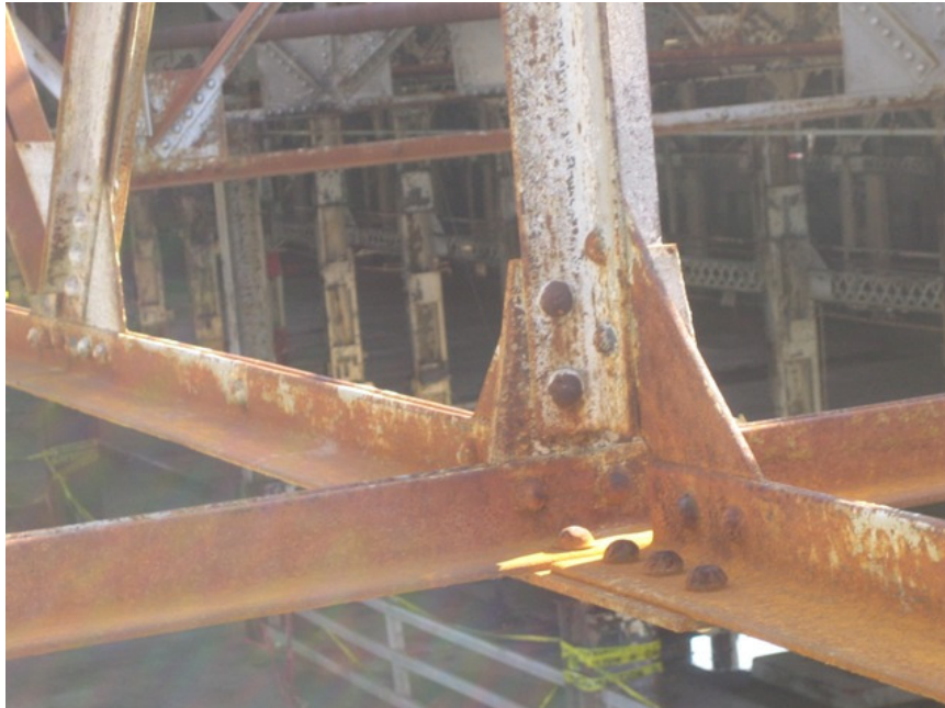
Photo #20: Typical rivet corrosion
