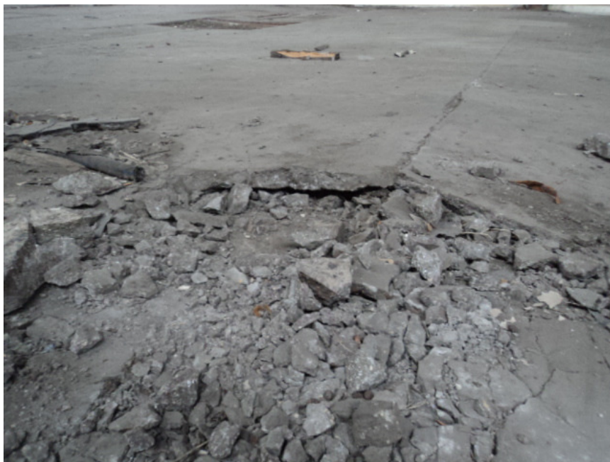
Photo #43: Slab-on-grade area of deterioration/damage
