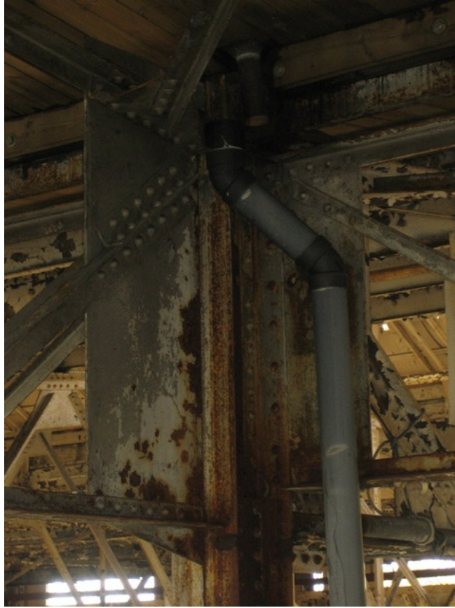
Photo #22: Typical storm water leader and corrosion at top of column
