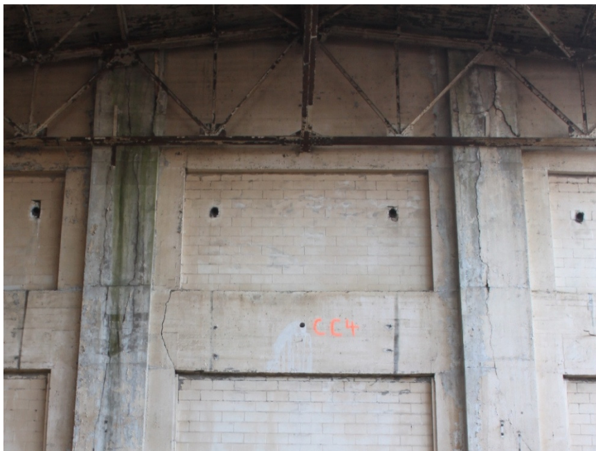
Photo #33: Exterior concrete wall deterioration
