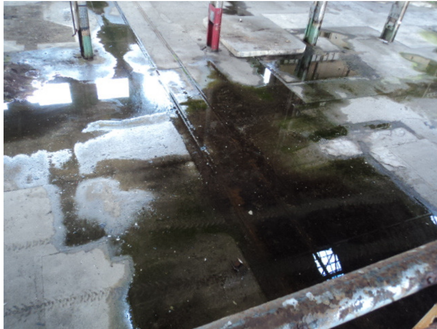
Photo #44: Slab-on-grade area of differential settlement
