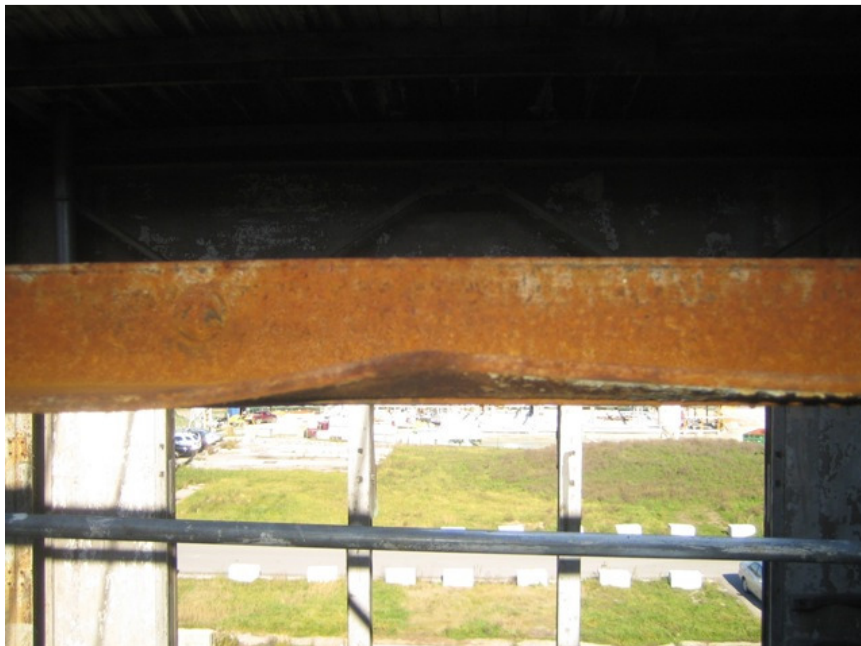
Photo #19: Typical dent/kink in truss member
