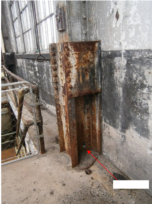
Photo #24: Burned hole through column web
