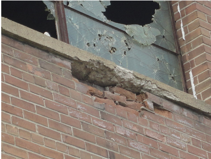
Photo #46: Typical deterioration of concrete sill and masonry below
