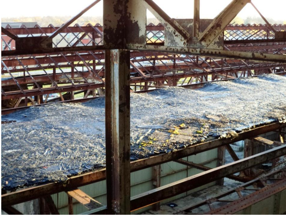
Photo #7: Typical Roof Deterioration
