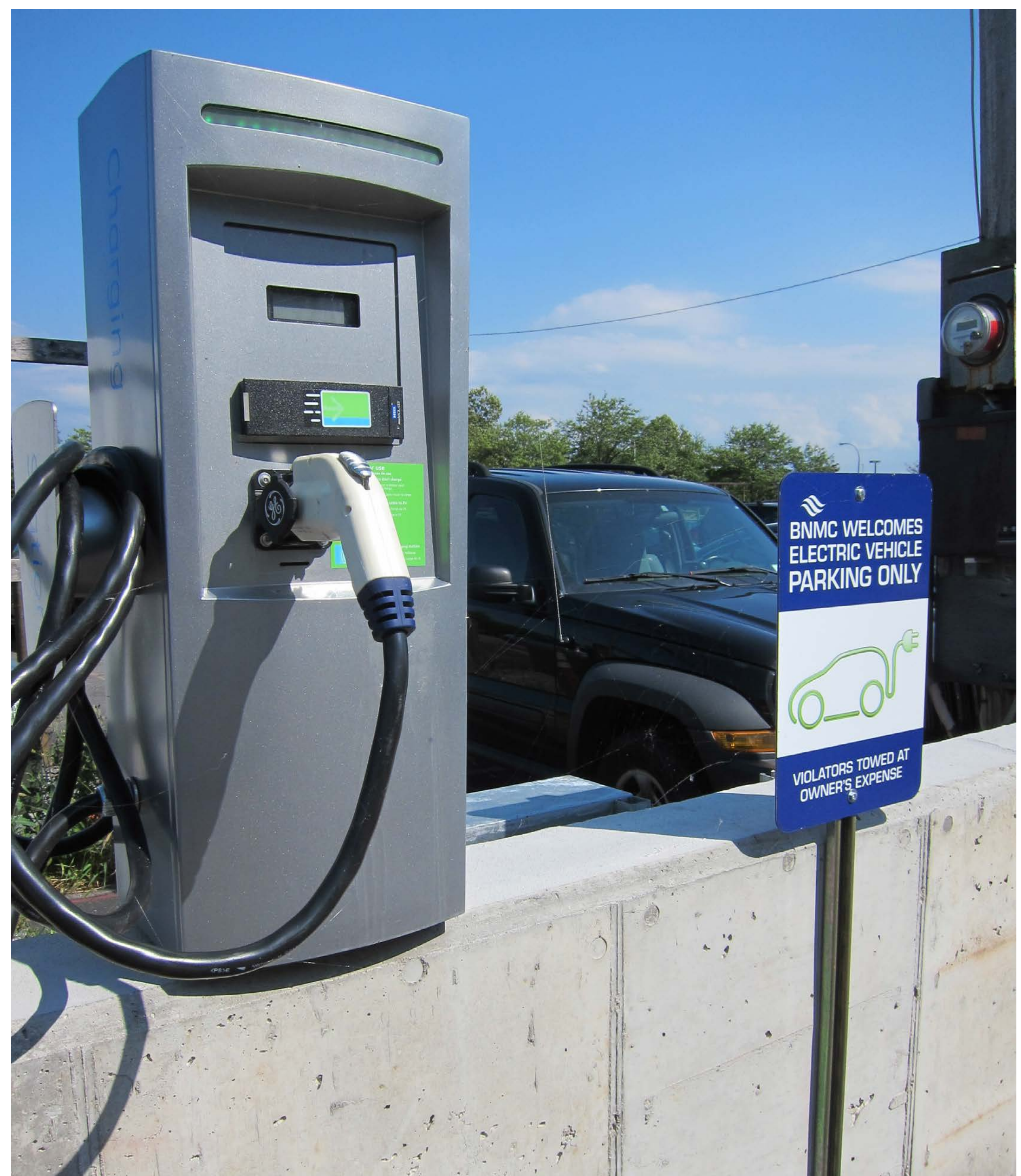
Electric car recharge station
